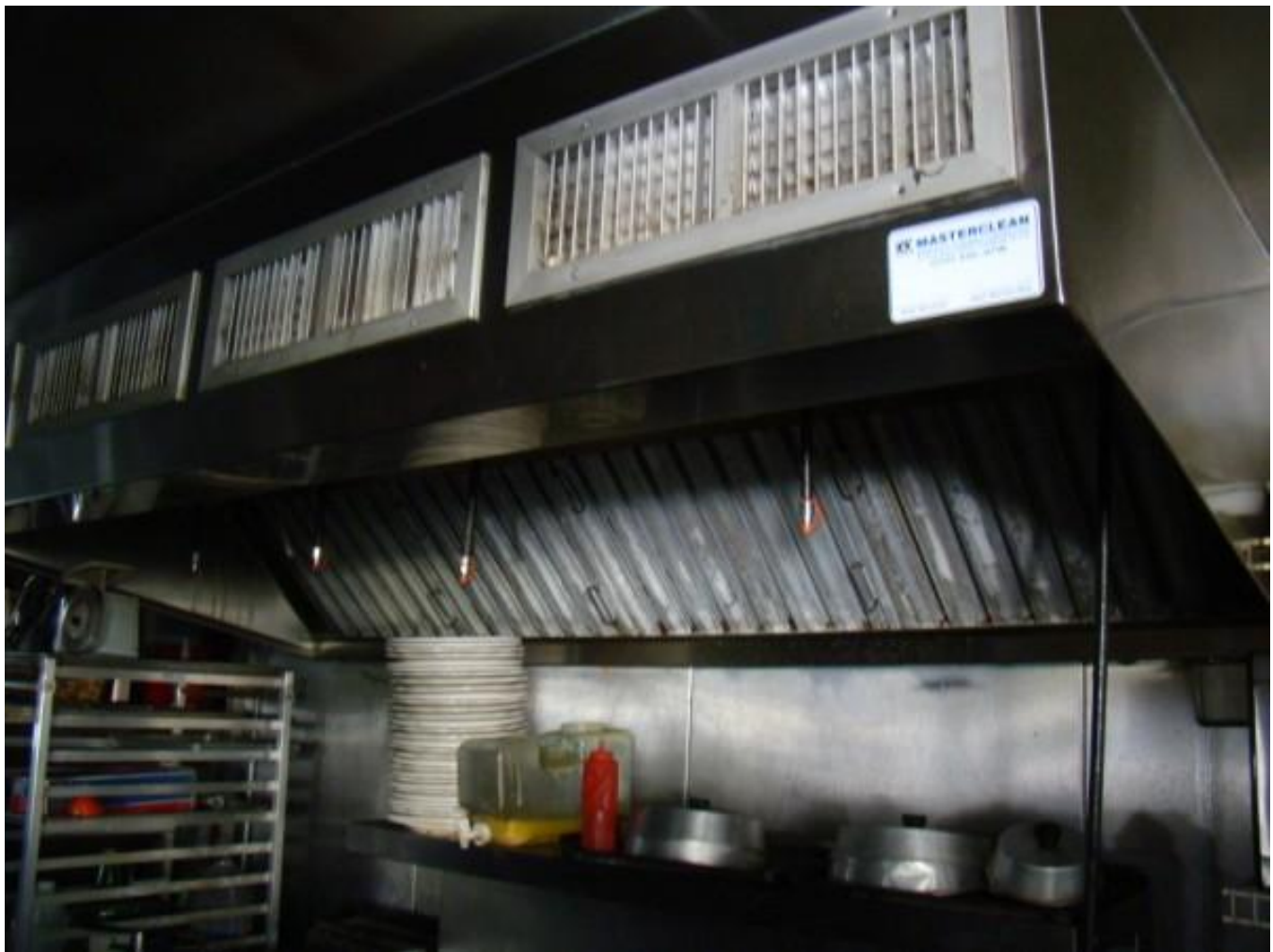
Hood w/ fire protection system – will be professionally removed before the auction
