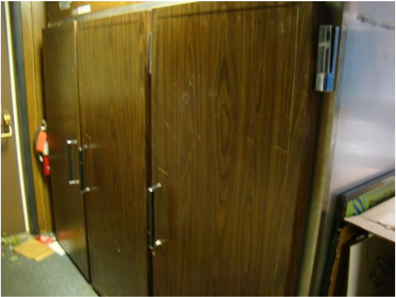
Reach-in refrigerator – top mounted compressor
